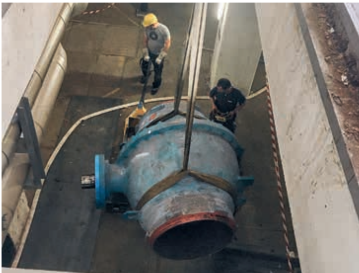
Removing a KHSVI ball valve after 25 years of use under difficult conditions
